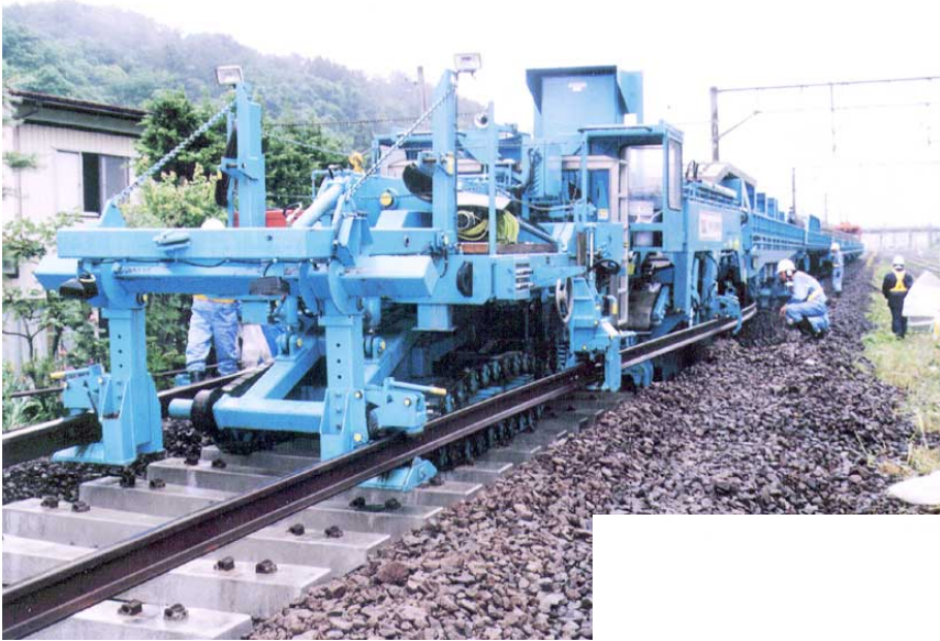
American track-renewal machine used for rebuilding to cope with limited construction period and workforce shortage (Jr East)
