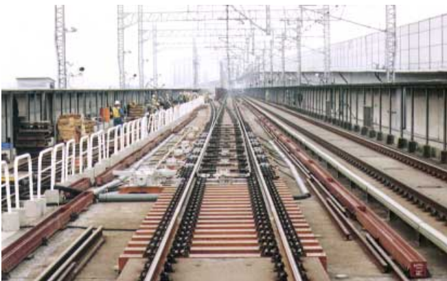
Hokuriku Shinkansen branches from existing Joetsu Shinkansen at this switching point 500-m north of Takasaki Station (JRCP)
